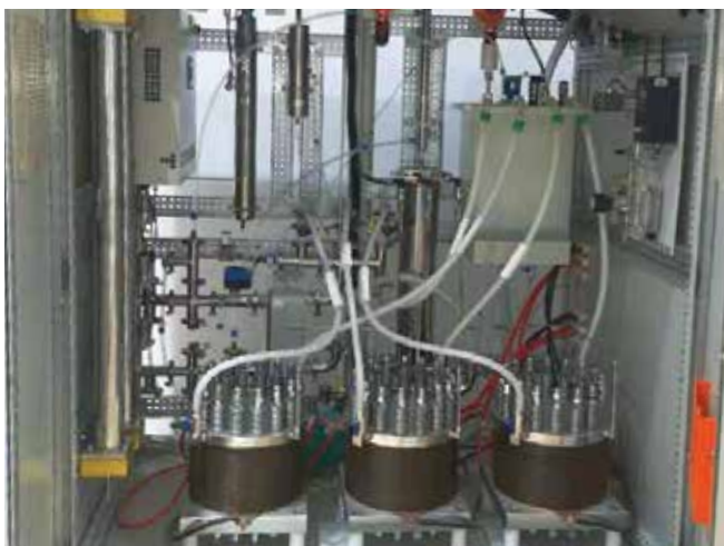
Electrolysis hydrogen production
